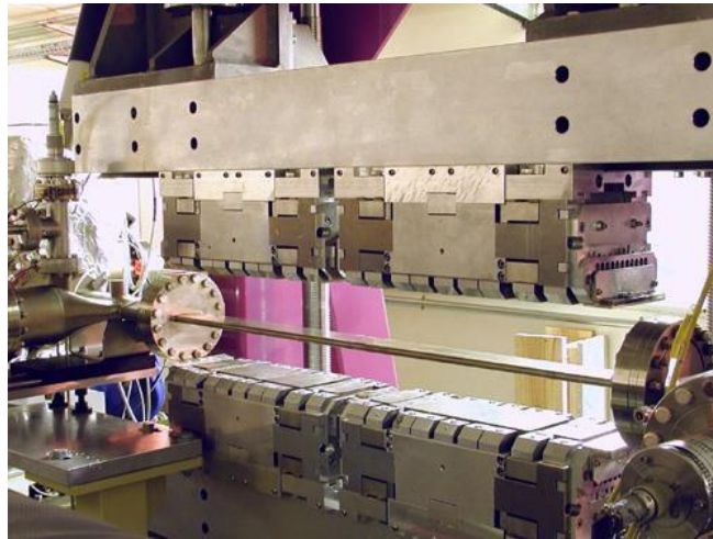
Figure 16: The 3 Tesla Asymmetric wiggler installed in the ID15 straight section
